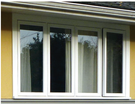
A comparison between a large single-pane fixed window with a narrow frame (above) and a sub-divided window with a wider frame, operable sashes and less glass area (below), illustrates how replacement windows can affect the appearance of a home.
