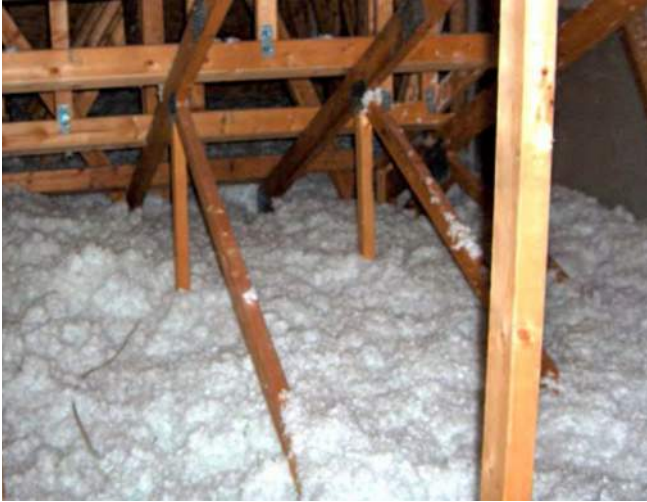
Blown-in attic insulation
