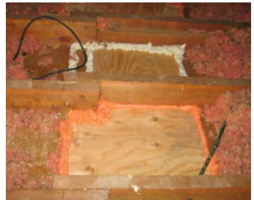
Spray foam around the edges of a cover, sealing it to surrounding joists and ceiling gypsum board.
