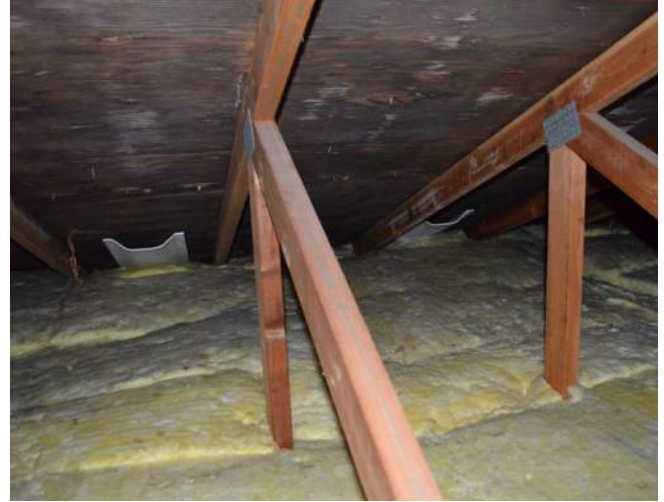
Insulation baffles installed at every second truss bay prior to installation of insulation to provide openings past the insulation from the soffit vents to the attic space.
