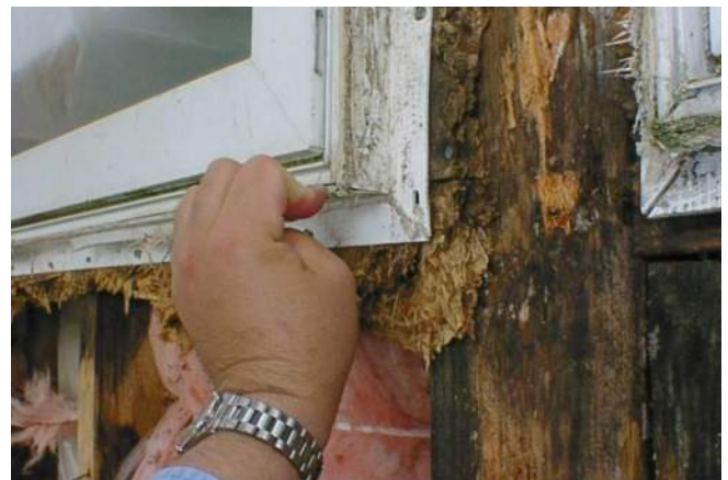
It may be desirable to replace windows and doors in cases where poor installations may have led to deterioration of the wall framing. The image above shows extensive decay visible at a window rough-opening interface detail upon removal of cladding. Damage extends well beyond window replacement work area.
