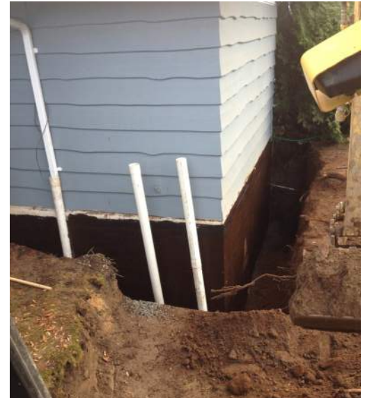
Adding exterior insulation to below-grade walls during foundation work is an effective way to increase the thermal performance of the wall.
