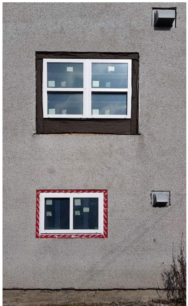
Windows being installed on a high wind- and rain-exposed facade with no overhang protection.
