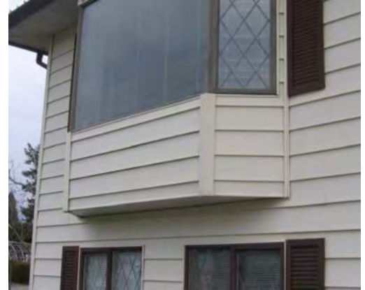
Overhanging floor under a bay window.
