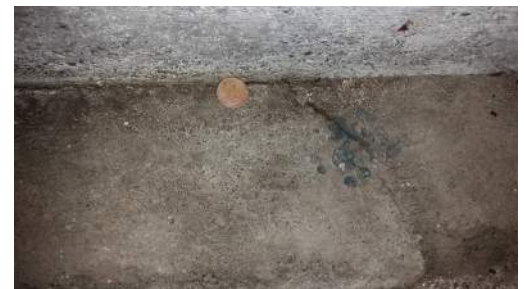
Cracks in the slab and gaps between the slab and the foundation wall.
