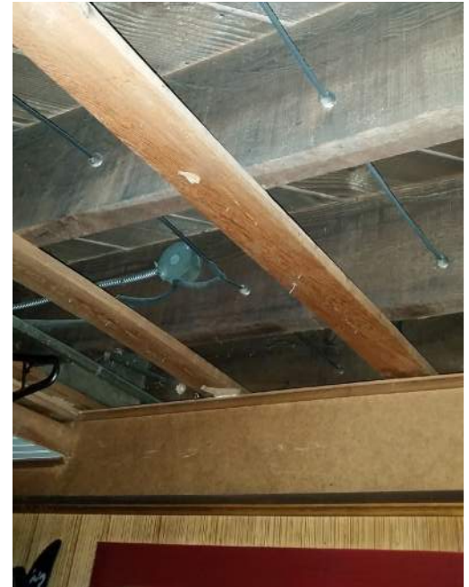
Non-insulated floor between a protected porch and a living space.
