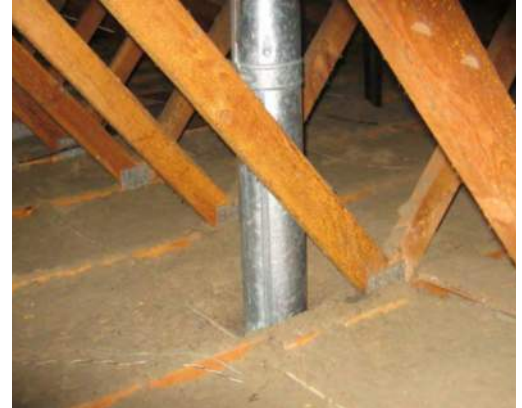
Uninsulated and un-sealed exhaust duct running through an attic, leaking air and heat to the space.
