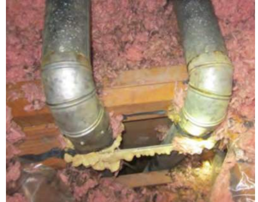
A relatively large hole in the ceiling plane through which two ducts are installed.
