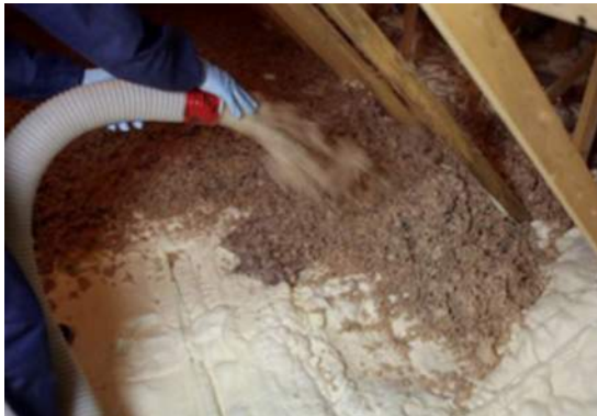
Insulation retrofit of an attic using blown-in cellulose added after air sealing and insulating with polyurethane foam.
