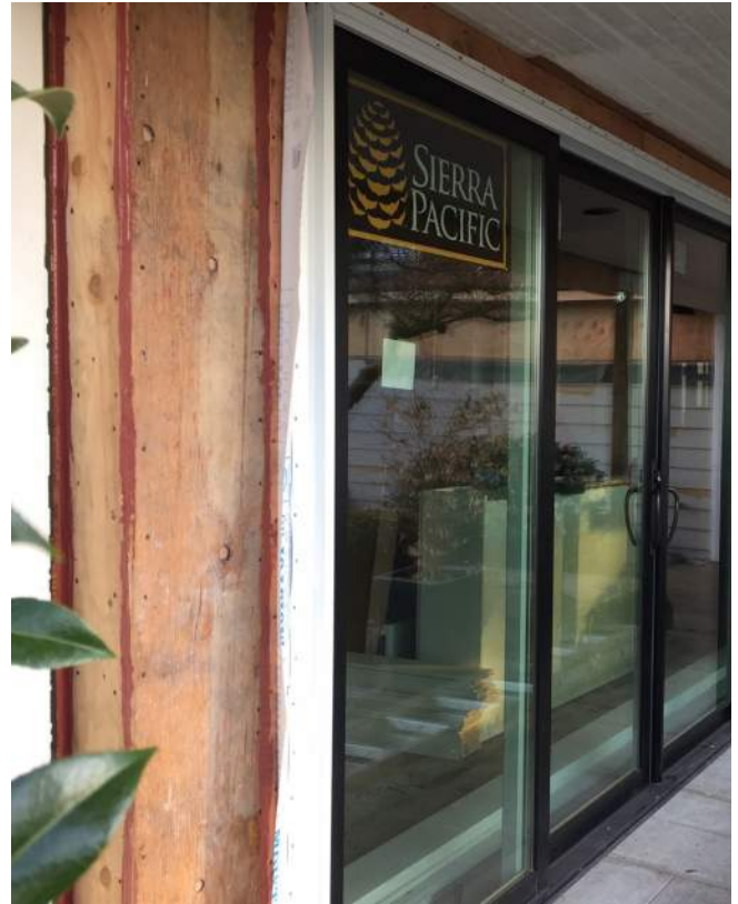
Replacement doors and windows are installed before the exterior insulation. For this project the air barrier approach was sealing all the gaps of the existing plywood sheathing.
