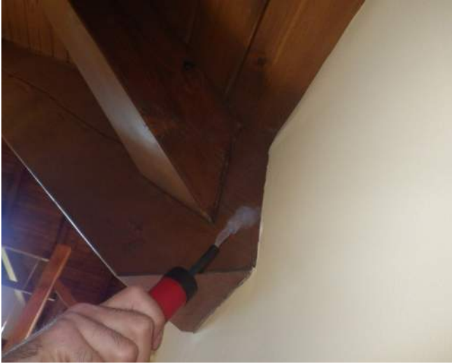
Smoke from smoke pencil being pulled through the wall indicating air leakage location.
