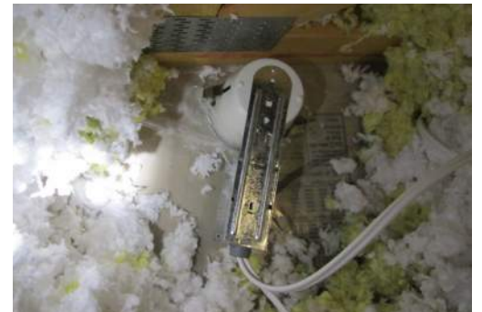
Above is an example of a poorly installed pot light where no measure of air sealing has been taken.
