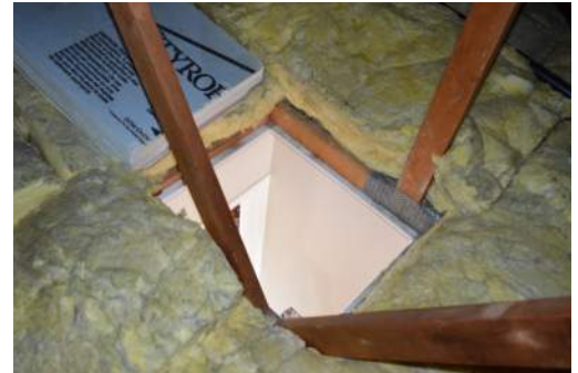
An access hatch with an insulated gypsum access cover.
