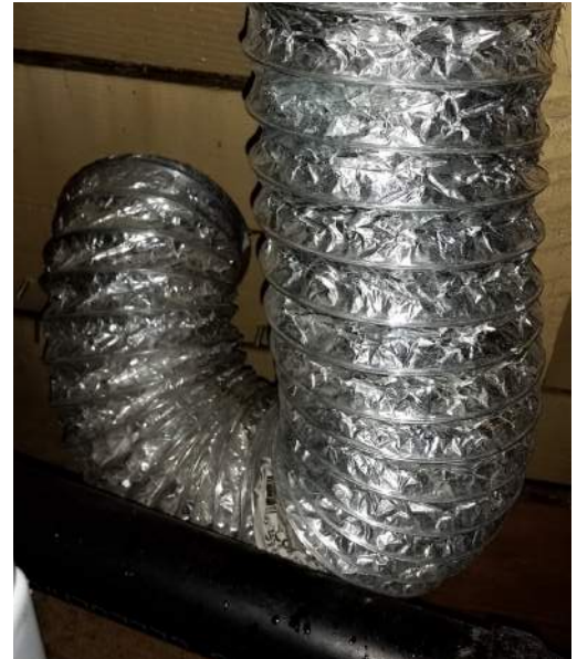
Unsealed duct penetrating the exterior wall. Duct penetrations should be airtight to avoid moist air being drawn through the wall and condensing inside the wall.
