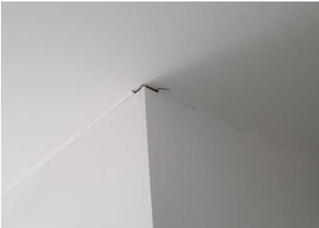
Visible crack on the interior finishes indicating possible air leakage location.
