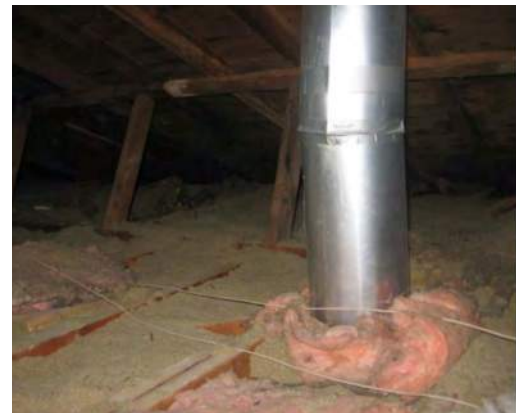
Insulated exhaust duct in attic.
