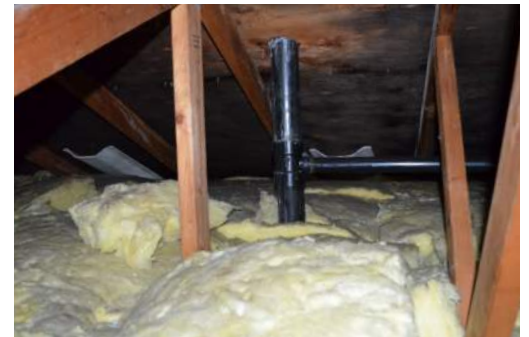
Accessible attic with potential air leakage around the plumbing stack penetration through the ceiling.
