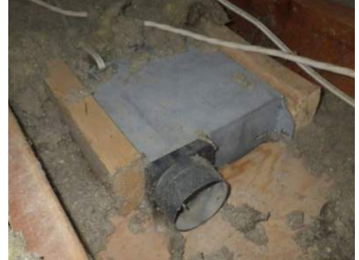
Bathroom exhaust fan venting into the attic. Conditions such as this should be remedied prior to or as part of air sealing and insulation work.
